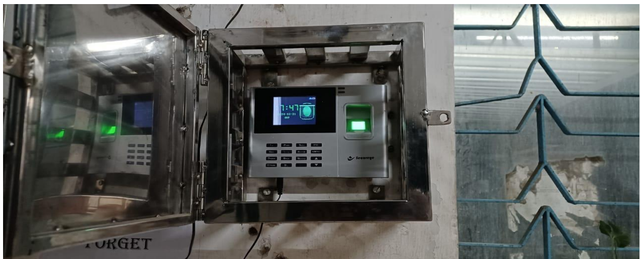
Installation of CCTV Footage & Biometric Machine
