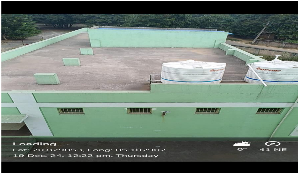
WATER STORAGE TANKS
